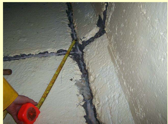
The west wall of the Kitsuksis Reservoir, showing signs of leaking
