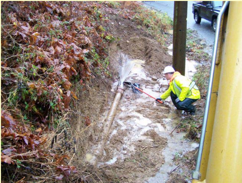
Broken watermain at Kitsuksis under repair
